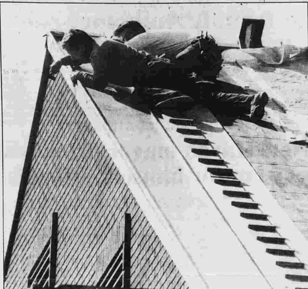
ROOF JOB — Bob Godden, left, and Ted Martin of C.G. Bostwick Co. of Hartford, lean against the roof of a building on Hartford Road Monday as they work to install a roof.
